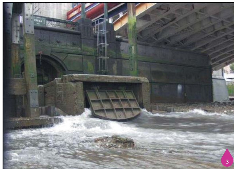
Figure 18.5: Brixton CSO discharging
