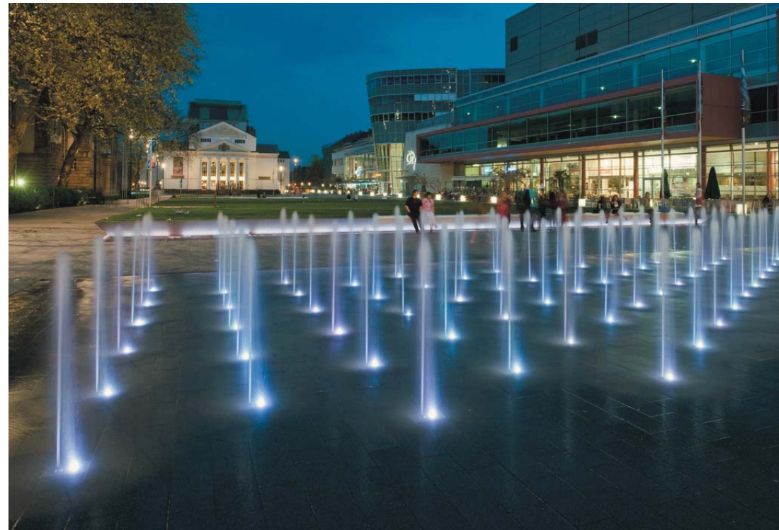
Figure 20.60: Example of lighting fixtures
