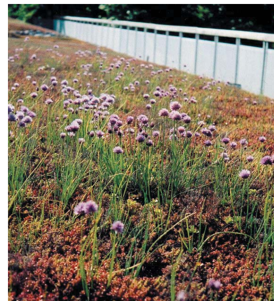
Figure 11.54: Brown roof planting
