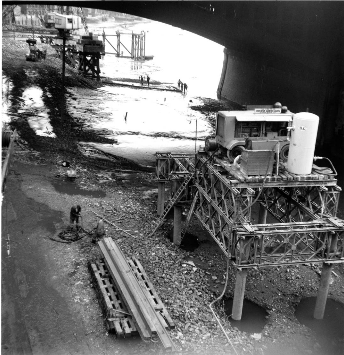
* A gantry (constructed as part of the Blackfriars Bridgehead Improvement Scheme) located on the foreshore in 1962; looking east beneath Blackfriars Bridge. 'Blackfriars Wreck 2' was discovered further to the east of this gantry, on the other side of the bridge; (Guildhall Museum 1962)
