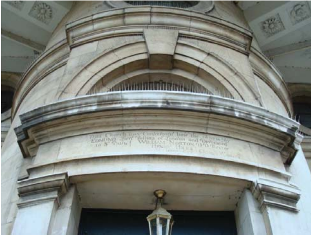
Stonework above western entrance showing opening of joints
