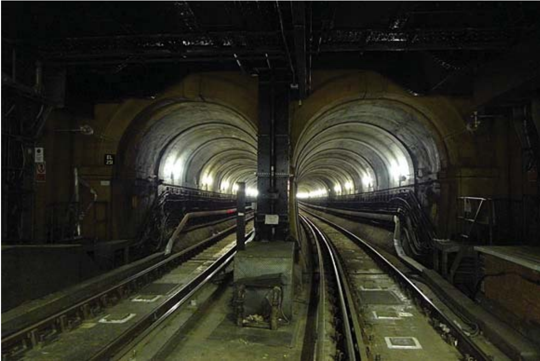
Vol 3 Plate E.99 The twin vaults of the Thames Tunnel viewed from the south
