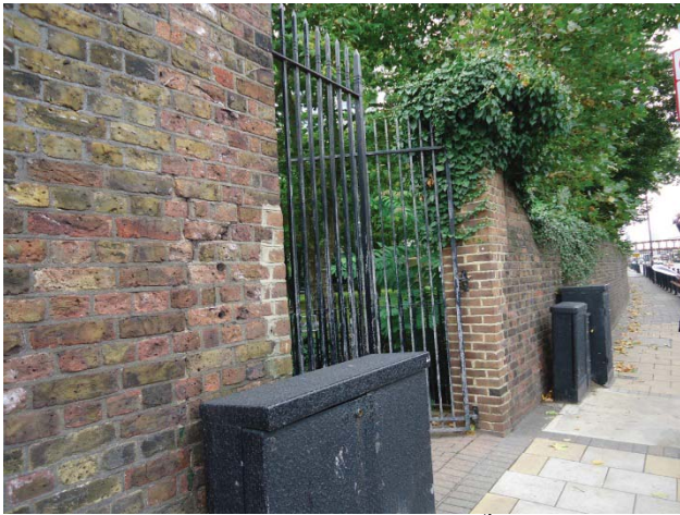
Caption 3: Eastern end of wall, showing 16 th century brick and vegetation growth
