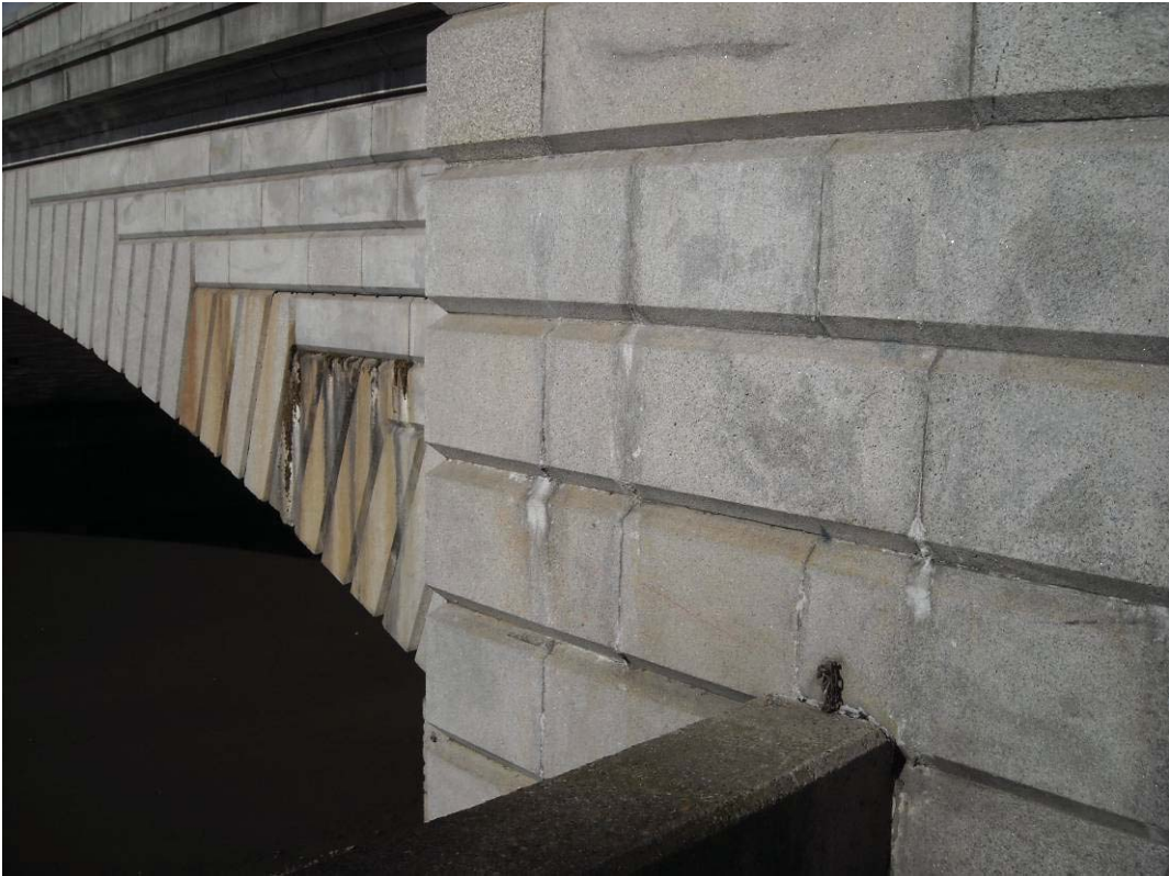
Vol 3 Plate E.10 Detail of north abutment and span 5 showing effects of leaching
