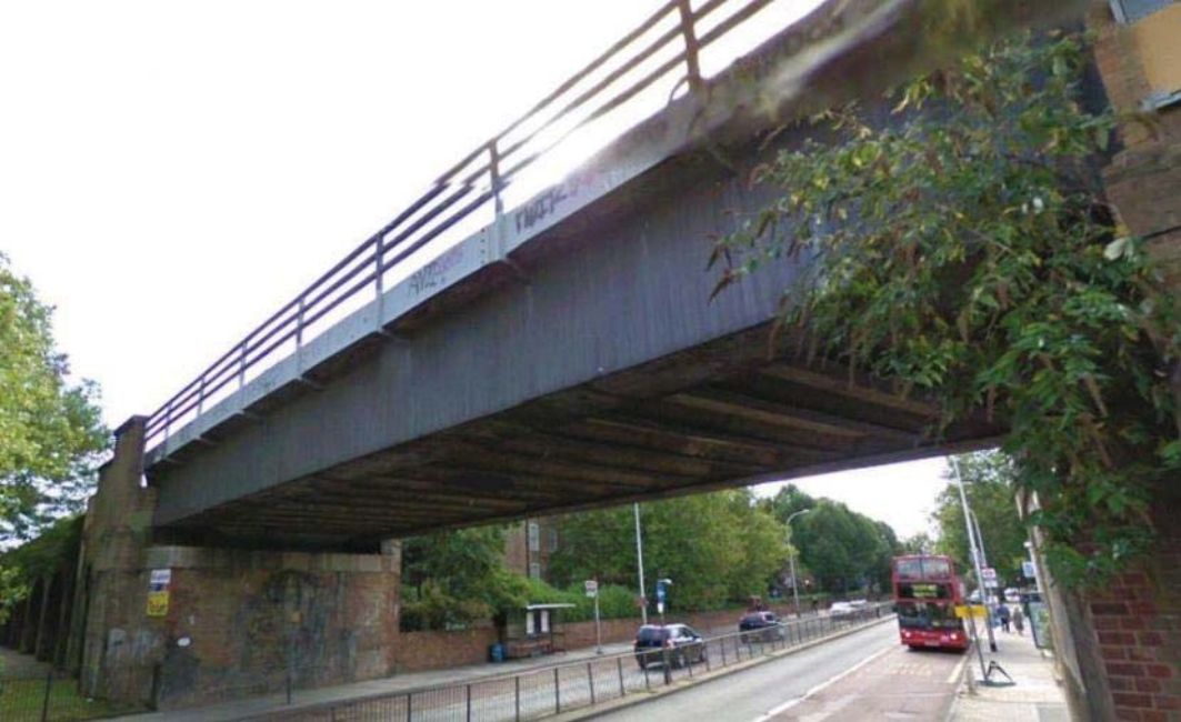
Vol 3 Plate E.124 Railway Bridge over Deptford Church Street viewed from north
