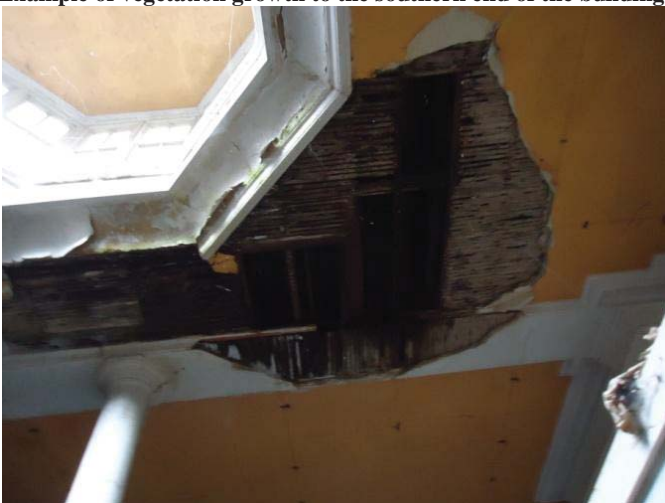
Damaged decorative features, and failure of lathe and plaster
