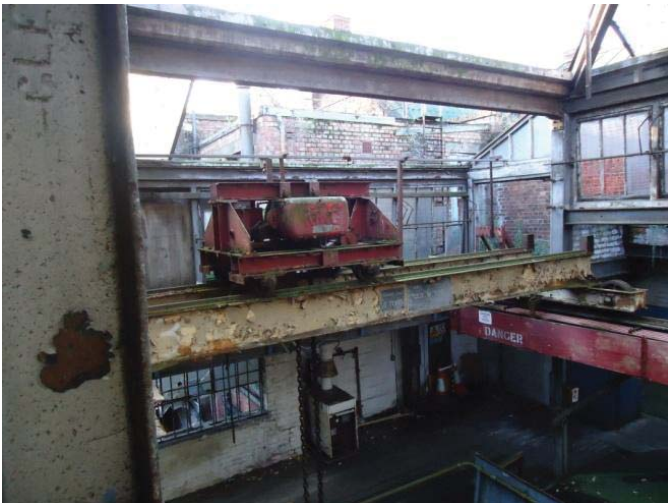
Example of retained machinery showing poor condition
