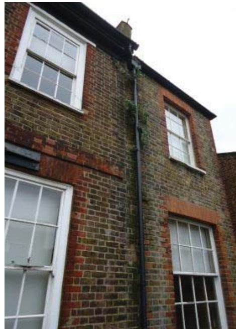
Water damage and vegetation due to faulty down-pipe
