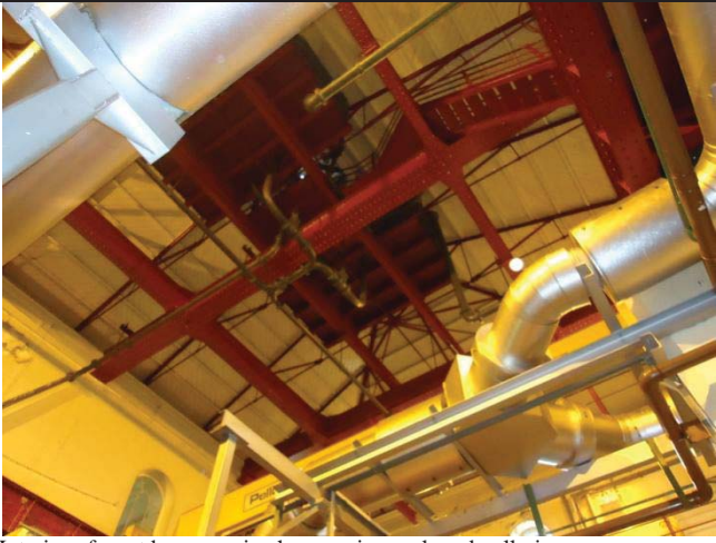
Interior of west beam engine house, pipework and galleries
