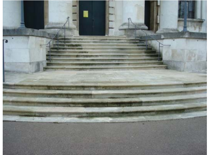
Western stairs showing wear
