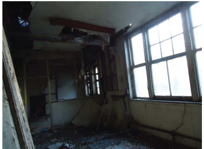
Interior of office range in poor condition
