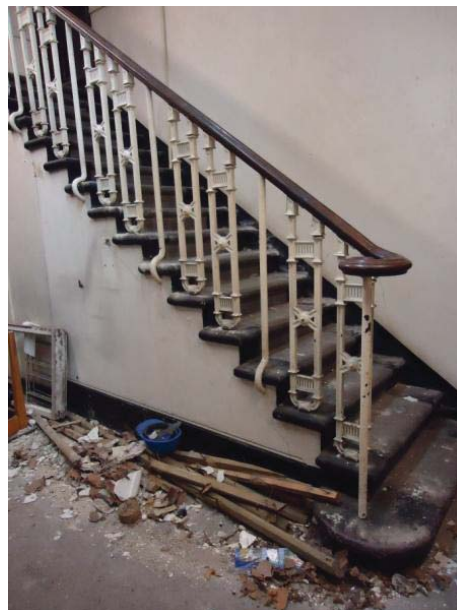
Main stair in neglected condition
