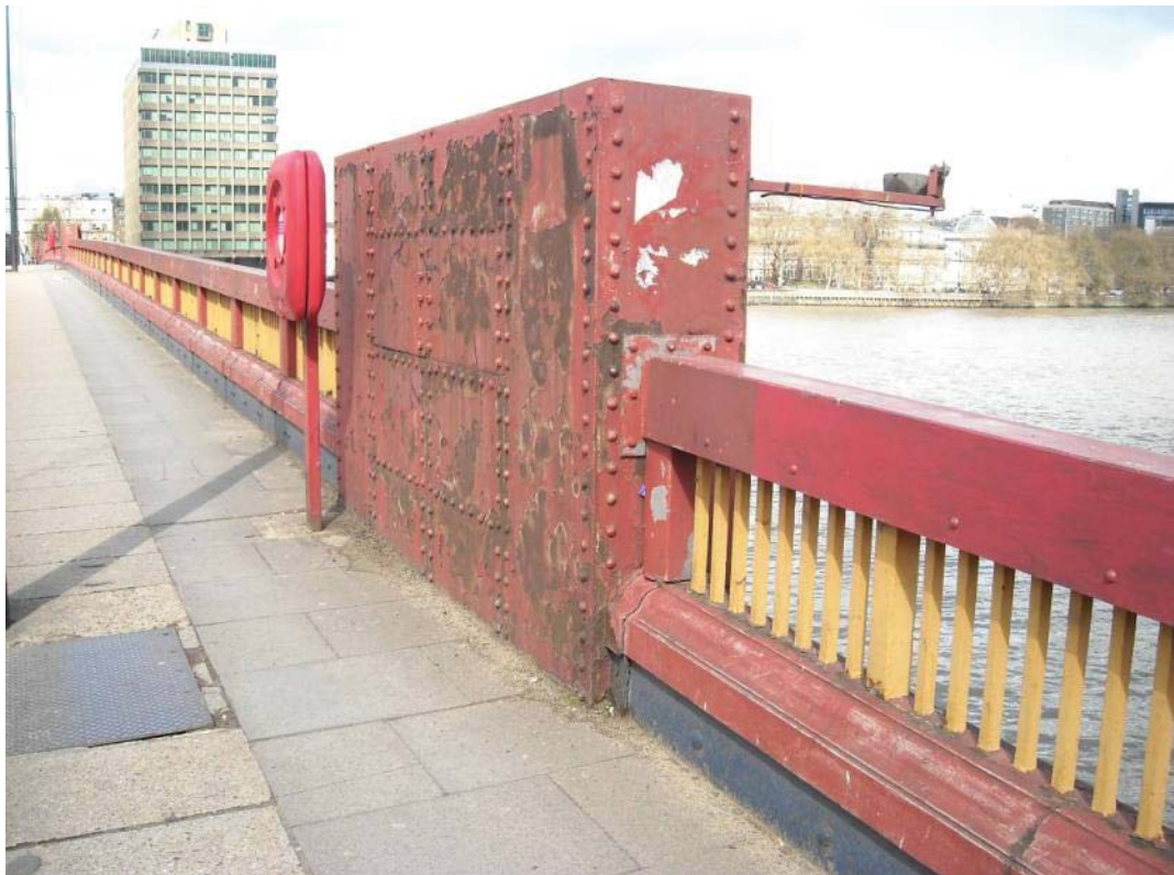
Vol 3 Plate E.58 East parapet showing typical failure of surface coatings & corrosion
