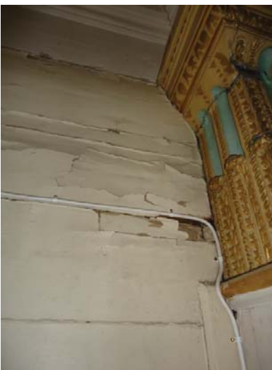
Detail of damage to plaster and decorative pilasters
