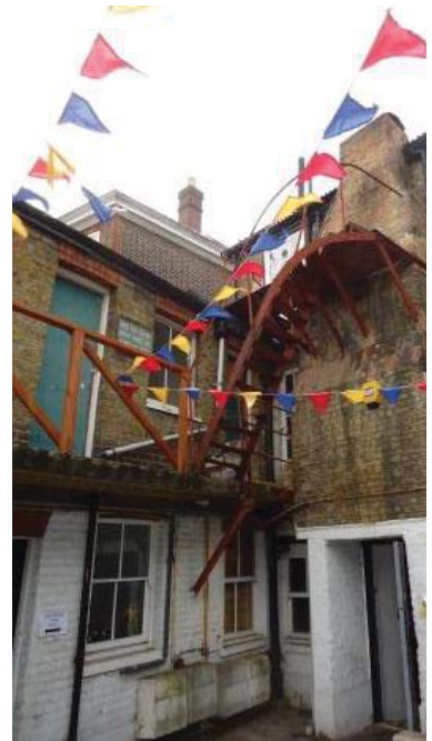
Iron stair to the rear of the building, in poor condition
