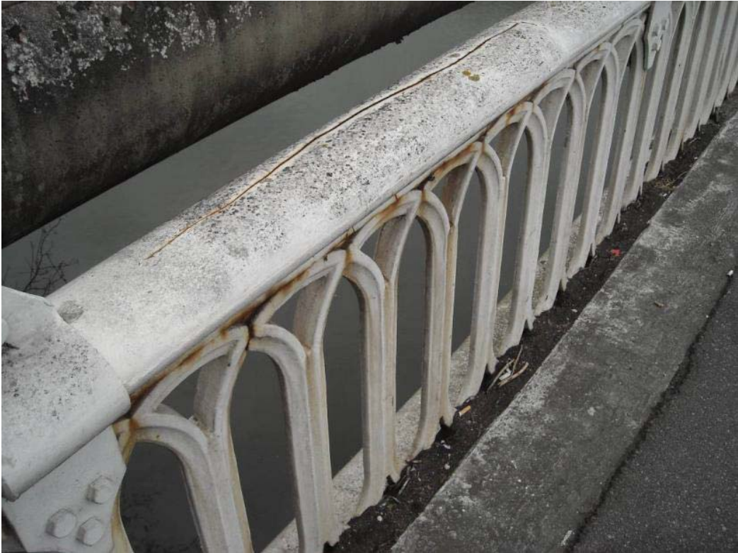
Vol 3 Plate E.134 Cast-iron balustrade and handrail, note cracking
