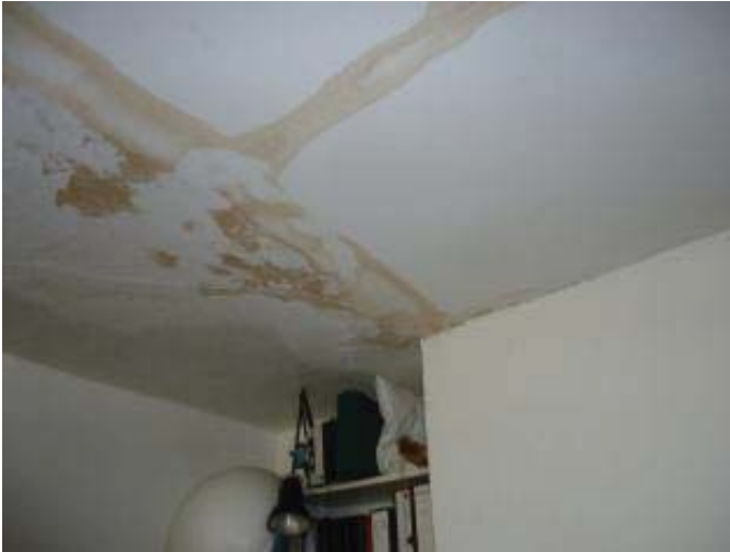
Example of internal water damage
