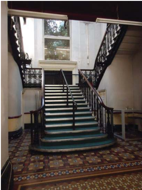
View of ground floor hall and main stair with wrought iron banisters
