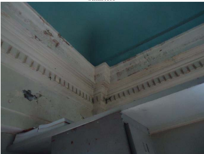
Damage from water ingress to the plasterwork of the main hall
