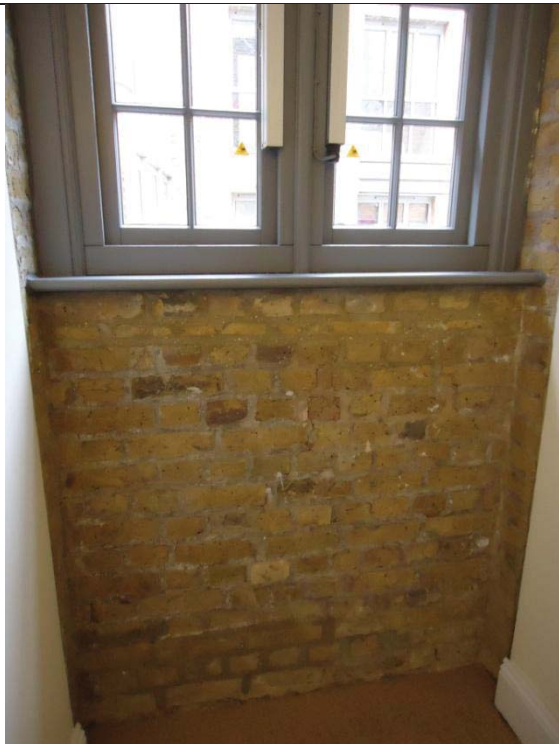
Small area of brickwork below southern window at each floor
