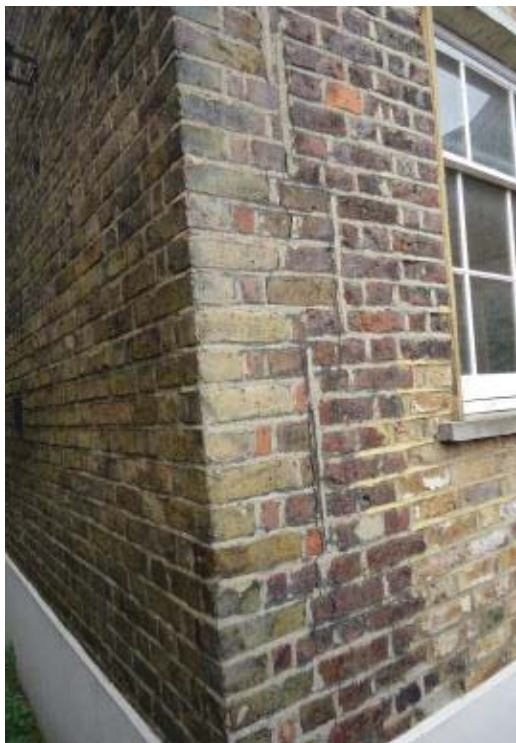
Example of cracking and poor brick repair
