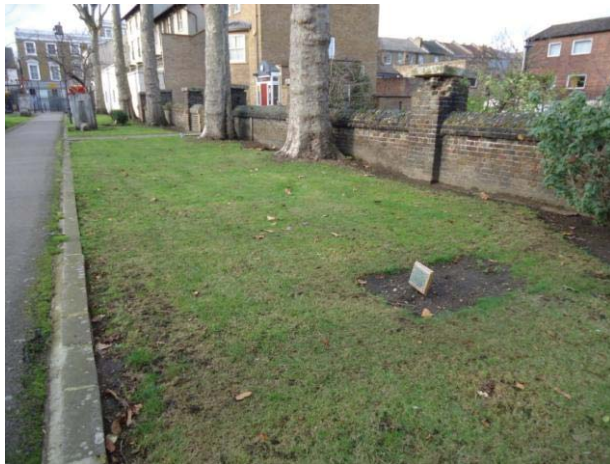
Boundary wall in poor condition
