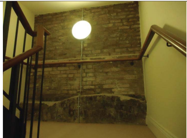
Evidence of arch, now filled in, west party wall (partially hidden by main stair)
