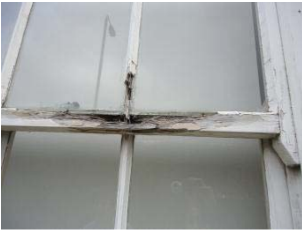
Example of degradation to timber sash windows
