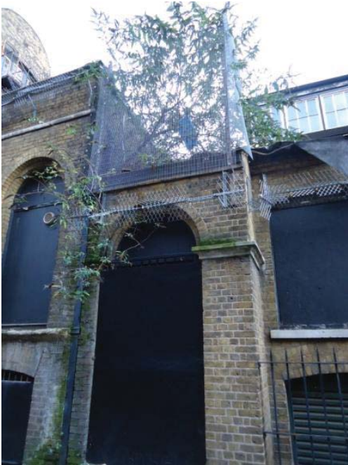
Example of vegetation growth to the southern end of the building
