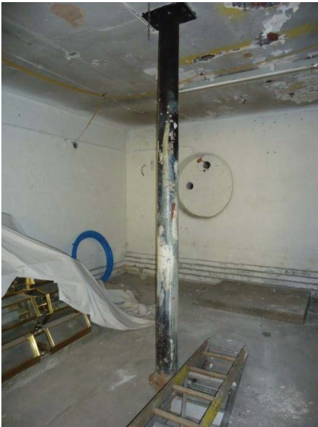
Internal cast iron column in basement – the pattern of columns is repeated throughout the building
