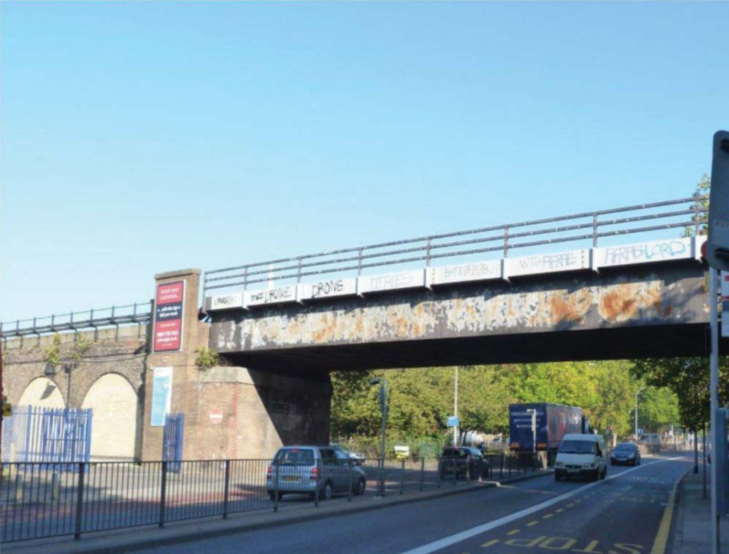
Vol 3 Plate E.123 Railway Bridge over Deptford Church Street viewed from south
