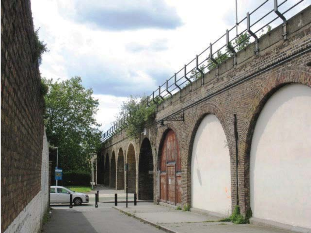
Vol 3 Plate E.105 View from Sun Wharf Viaduct towards Browne House and Farrer House Viaduct
