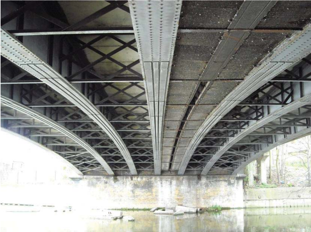
Vol 3 Plate E.132 Underside of west span, with 1990's strengthening plates to girders
