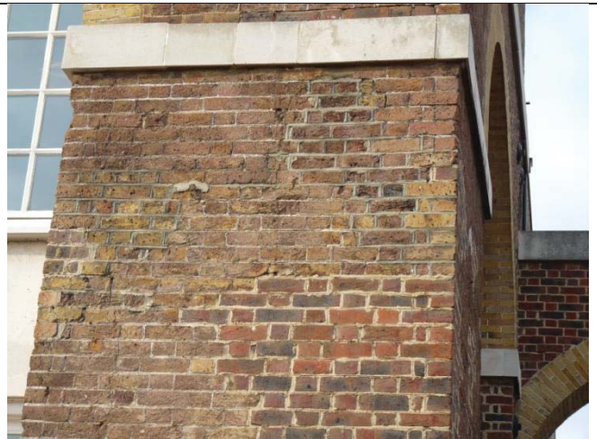
Example of variously coloured brickwork in poor condition
