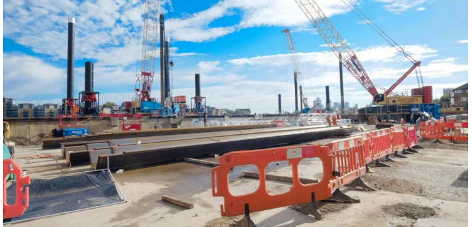
Chambers Wharf in Bermondsey preparing for the installation of the sheet piles for the cofferdam
