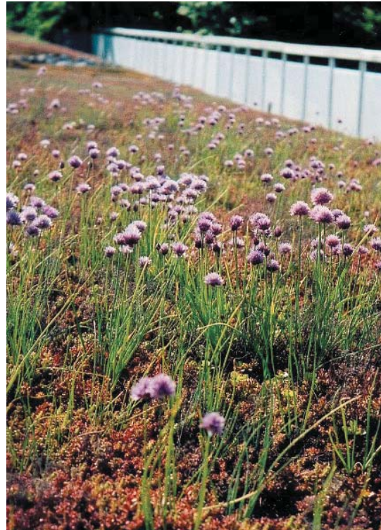
Figure 12.49: Example of Brown roof
