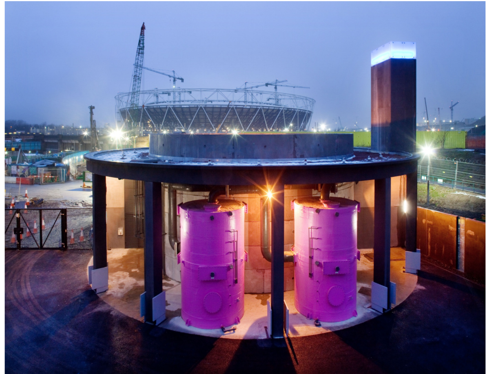
Figure 4.1: Example of good design in recent Thames Water projects at Pudding Mill Lane Pumping Station on the Olympic Site (Source: Olympic Delivery Authority)
