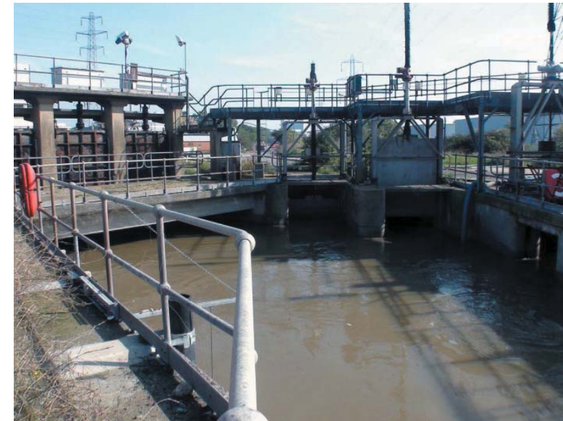
Figure 28.10: Inlet to the treatment works from the northern outfall sewers
