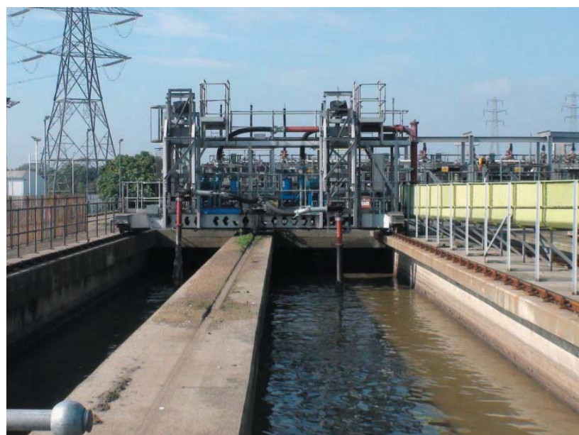
Figure 28.7: Existing grit channels and gantries
