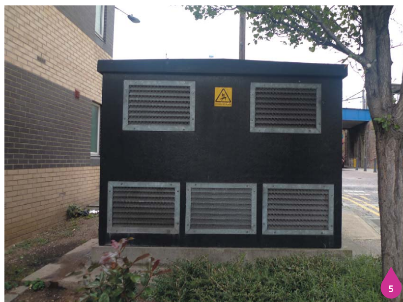
Figure 29.7: Existing Electrical sub-station on Bekesbourne Street
