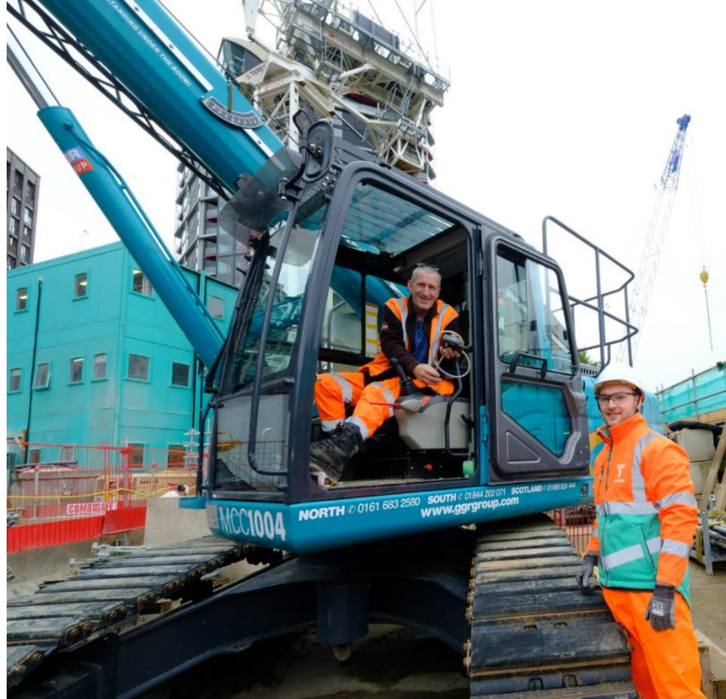
EU Emissions stage 5 crane used to lift the workforce into the CSO shaft
