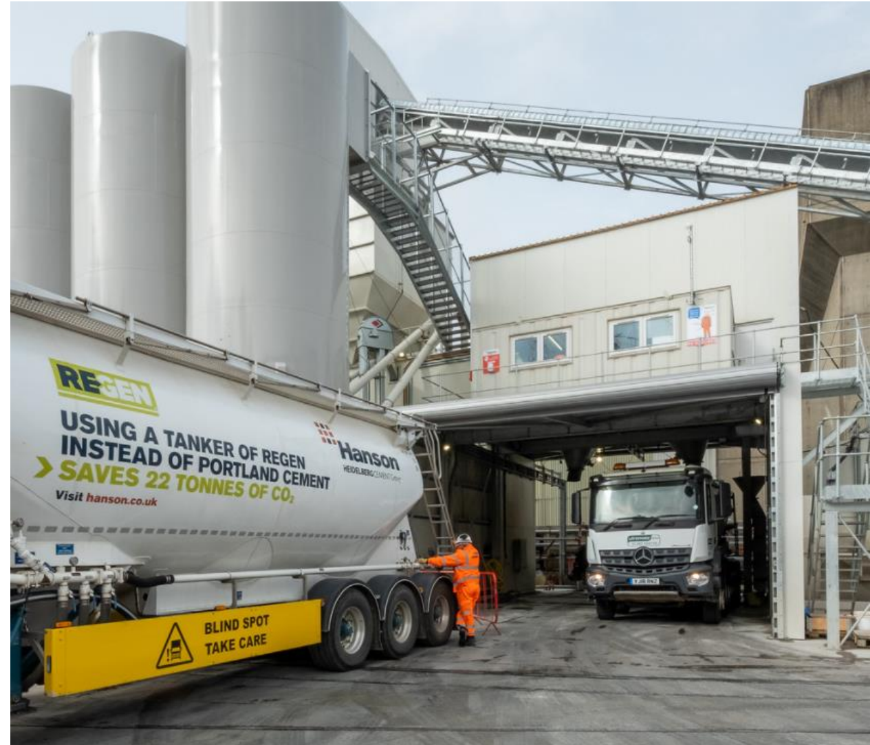
Low carbon cement delivery at the acoustically clad on site concrete batching plant
