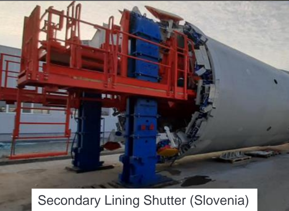
Secondary Lining Shutter (Slovenia)
