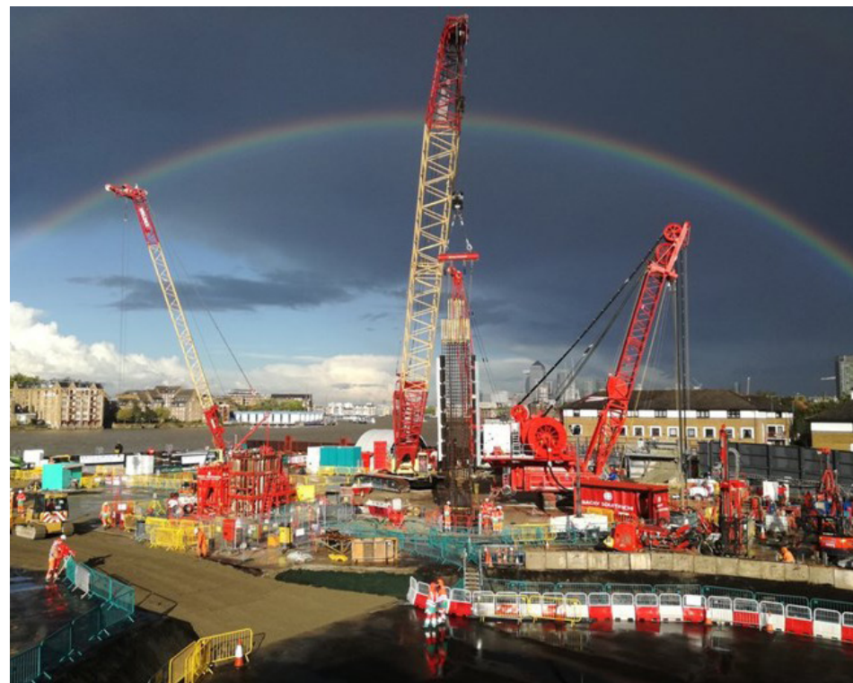
An innovative, electrically-powered hydrofraise diaphragm walling machine was used to help build the Thames Tideway Tunnel
