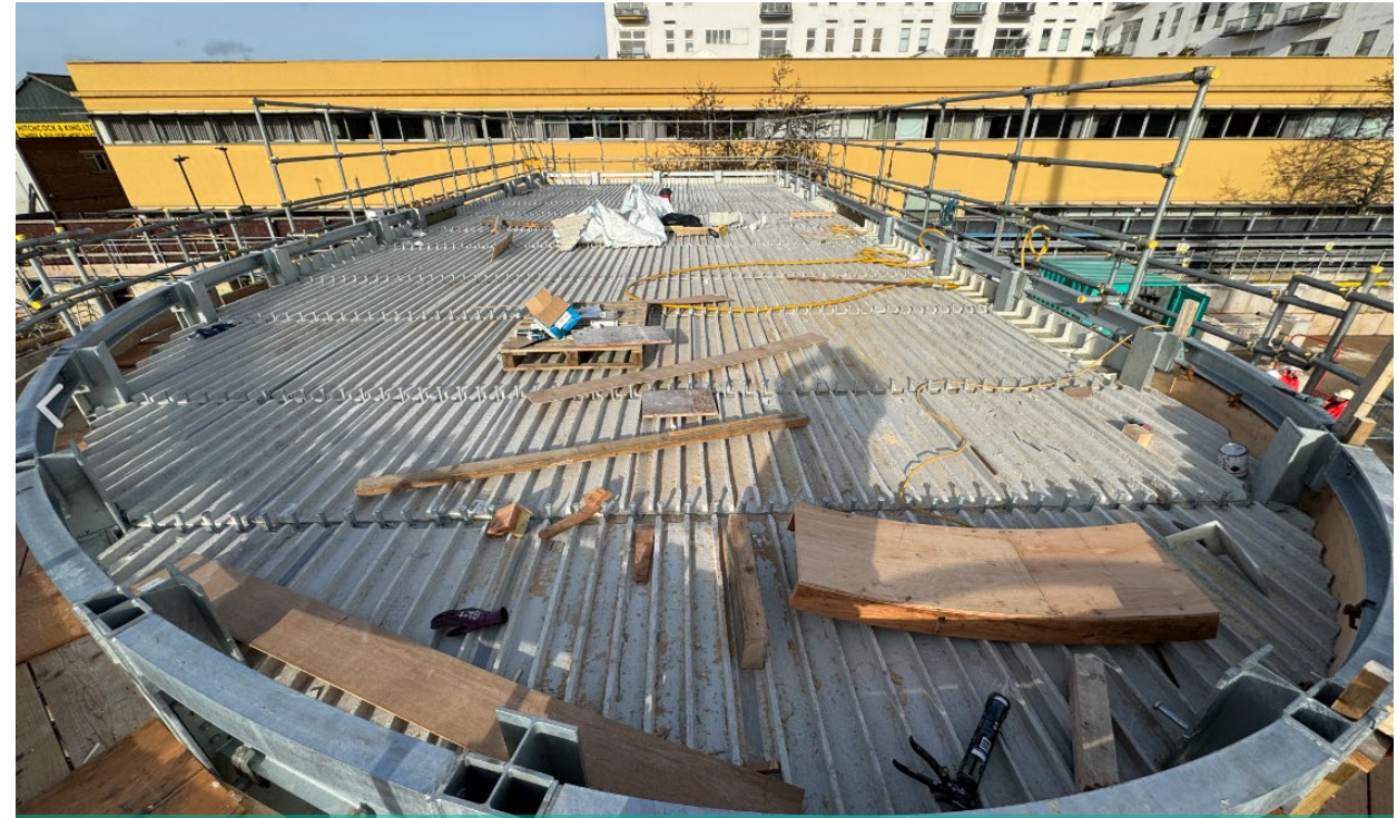
Mechanical and Electrical Kiosk Install external cladding and doors and installation of brown roof
