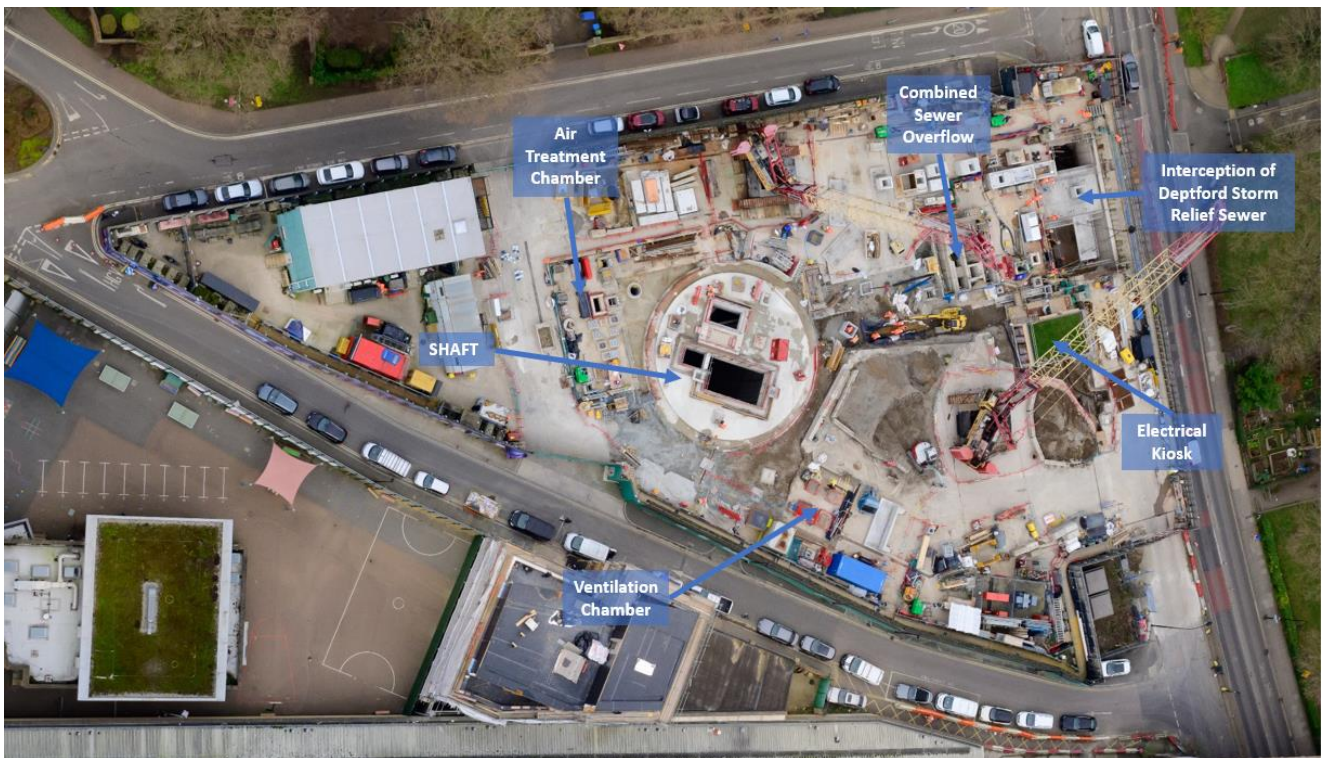
An aerial photograph taken in January 2024 which shows the current areas of construction
