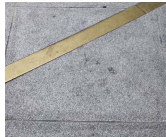
Figure 17.57: Example of metal fleck in paving
